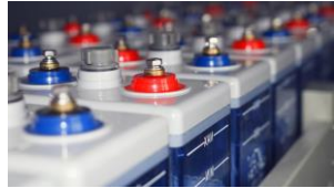
Energy Storage & Batteries
